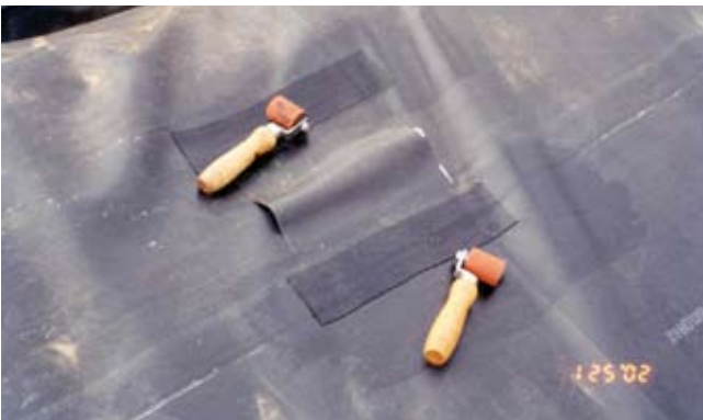
Figure 10E-29 Covered liner vent
