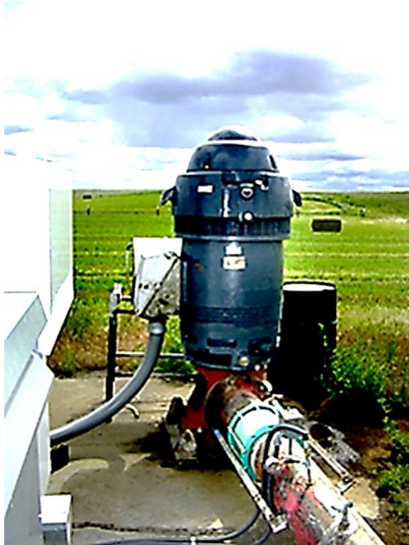
Figure 650L-43: Water well pump image powered by electric motor, Washington
