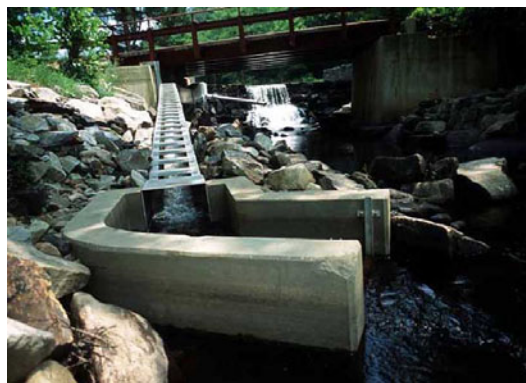
Figure 611–3 This fishway was funded in part by the NRCS-WHIP program to provide passage to spawning habitat for migratory fish (photo courtesy Paul Fusco, USDA NRCS)
