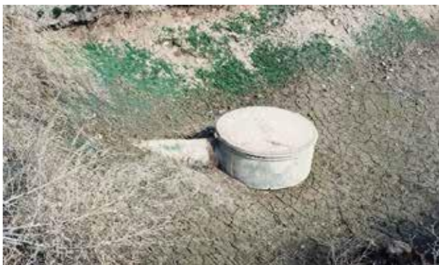
Figure 8B–1 Suction end screen with internal spray Twin Falls, ID
