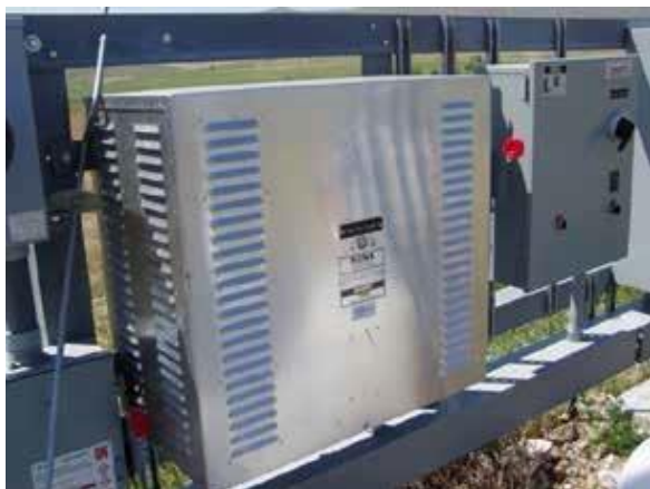
Figure 8–63 Static-phase converter center-pivot irrigation system near Ellensburg, WA
