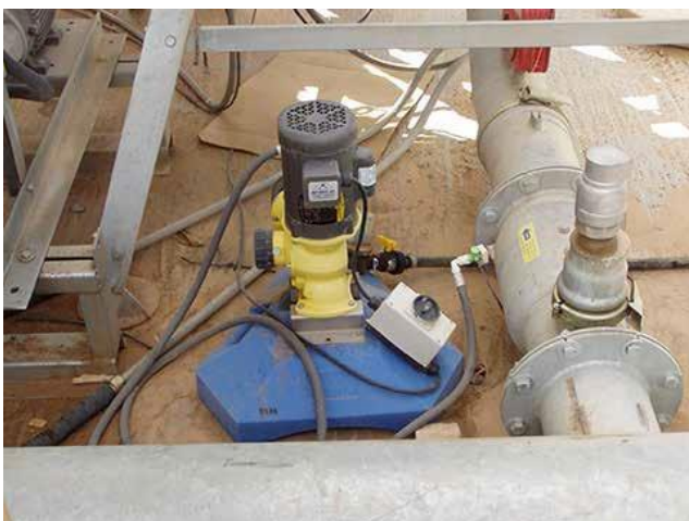
Figure 8–50 Diaphragm pump primer used for chemigation on a center pivot
