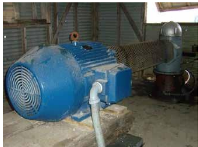
Figure 8–91 Electric motor powering a turbine pump at LSU Rice Research Station near Rayne, LA
