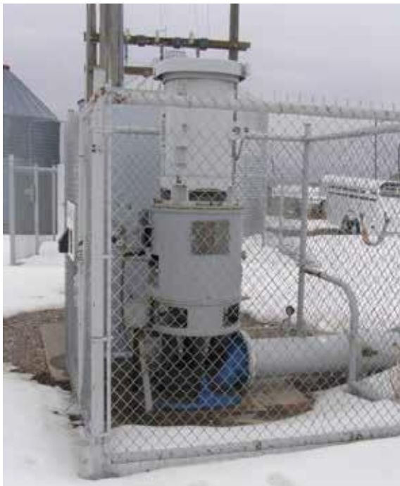
Figure 8–58 Vertical magnetic drive, A & B Irrigation project near Rupert, ID
