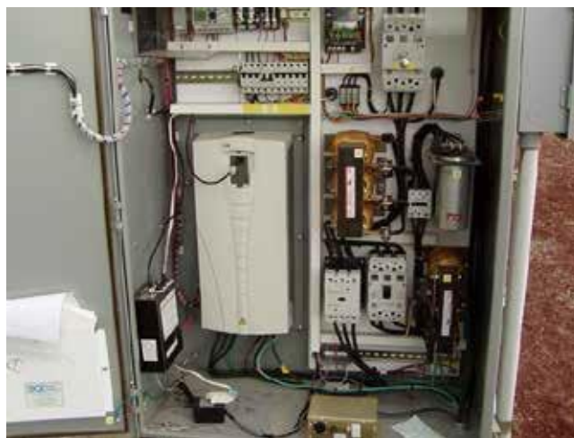
Figure 8-89 Variable-frequency drive and pump panel near Nampa, ID
