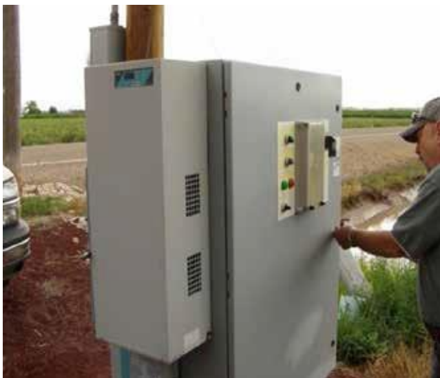
Figure 8-93 Pump control panel near Nampa, ID
