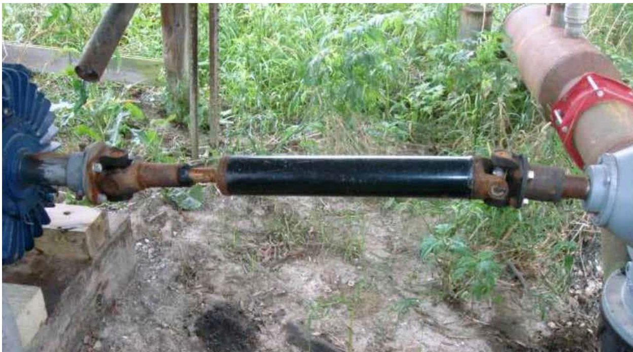
Figure 8A–6 Electric motor hooked to a 90-degree angle gear drive, Vermillion Parish, LA
