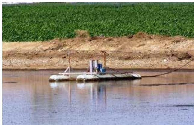
Figure 8–29 Pump unit on a floating barge in an animal waste pond near Nampa, ID
