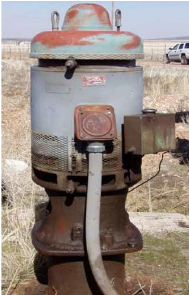
Figure 8–101 Oil-lubricated deep-well turbine pump near Flowell, UT
