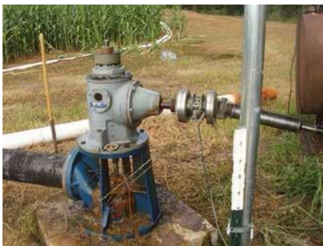
Figure 8A–4 Torques cell installed to measure engine output horsepower during Louisiana NRCS pumping plant evaluation
