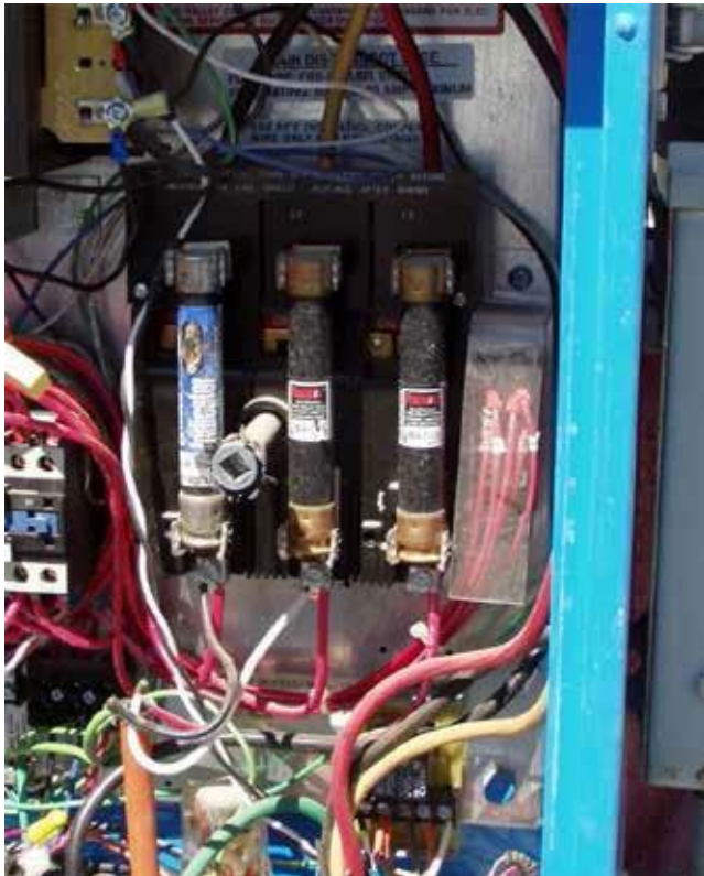
Figure 8–83 Fuses installed in a control panel
