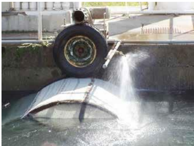
Figure 8B-4 Rotating screen with external spray near Boardman, OR
