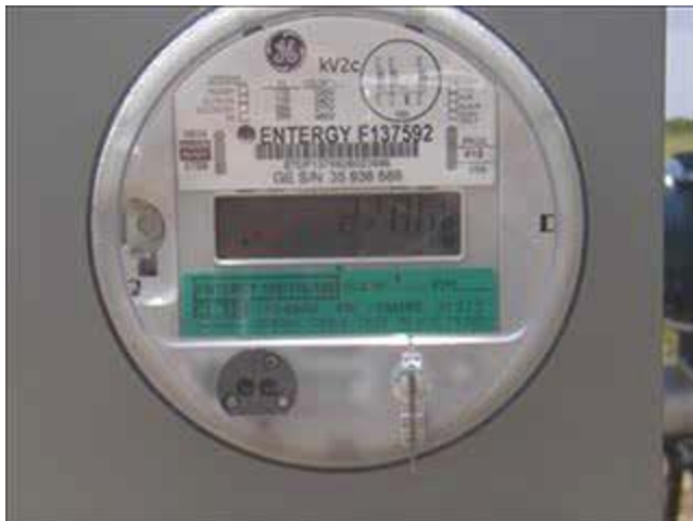
Figure 8A-2 Programmable electric meter red oval surrounds area with flashing indicators.
