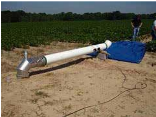
Figure 8A–5 Discharge pipe with flow meter and valve
