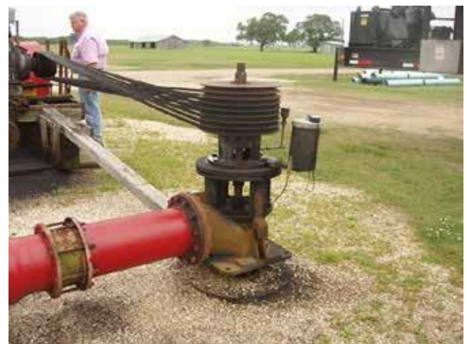
Figure 8-56 Turbine pump with V-belt drive south of Crowley, LA
