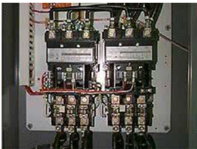
Figure 8-77 Pump starter and overloads (courtesy of the Irrigation Association)
