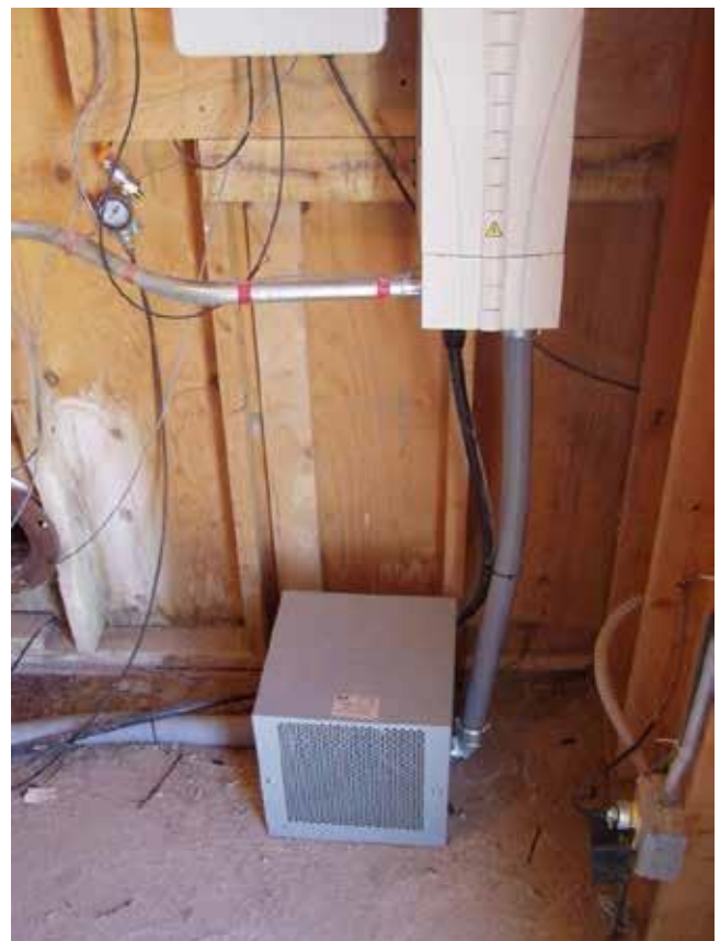
Figure 8–90 Variable frequency drive with input line filter near Kimberly, ID
