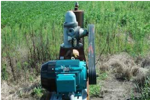
Figure 8–96 Belt drive with belts exposed for inspection
