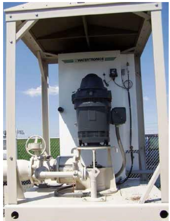
Figure 8–61 Pump and pump shade near Othello, WA
