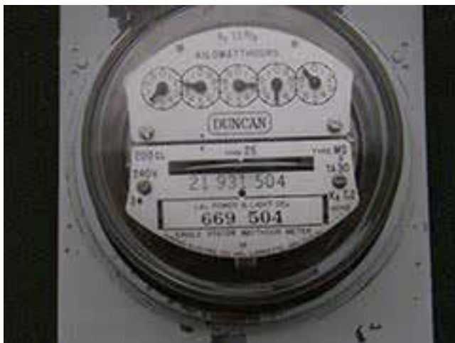
Figure 8A–1 Front of electric meter showing K_h factor
