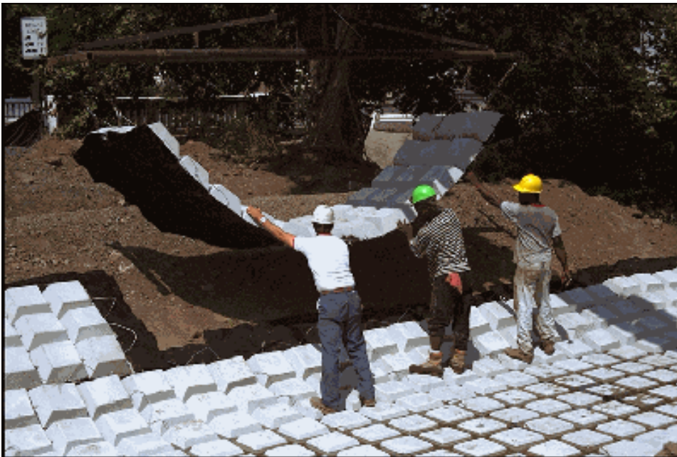
Figure 44: Installation of an ACB Lining With Geotextile Attached – Not Recommended
