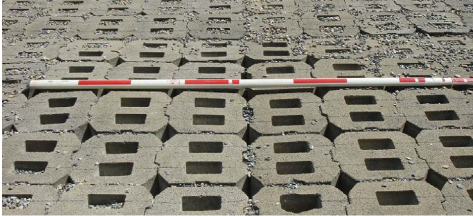
Figure 50: Depression Observed in ACB Surface
