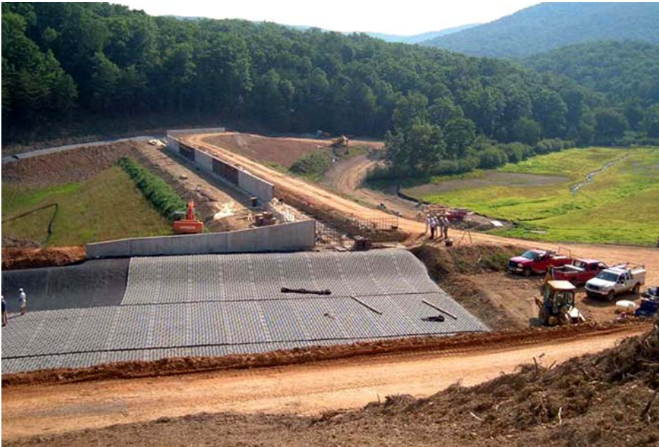
Figure 1: ACB-Lined Spillway (NRCS-VA)
