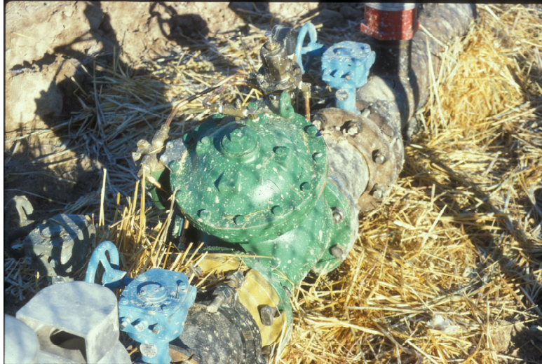
Figure 4-42 A hydraulic control globe type pressure reducing valve on an irrigation mainline
