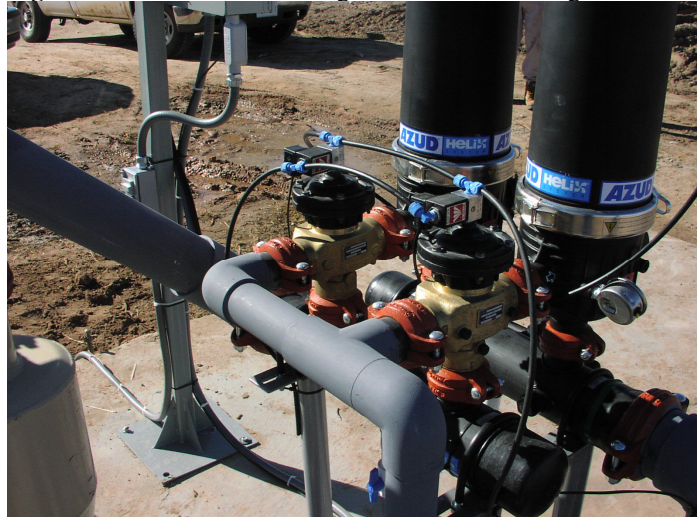
Figure 4-44 Pressure sustaining valve on a microirrigation filtering station
