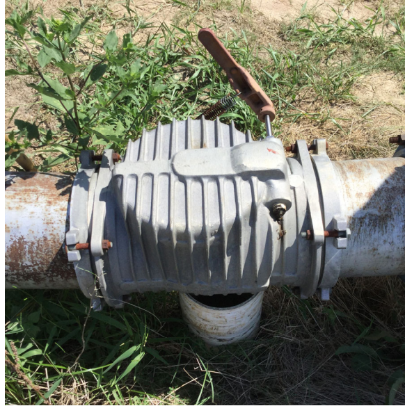
Figure 4-46: Check valve installed on a pumping plant
