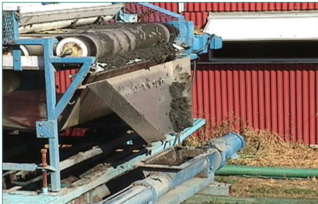
Figure 4–12 Belt press (Texas A&M AgriLife Extension Service)
