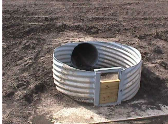
Figure 13-44: CMP Riser with Stoplogs
