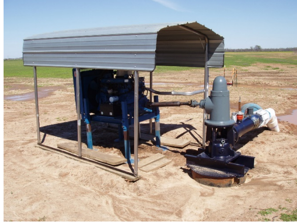
Figure 13-24: Hydrology Enhancement with Pumped Ground Water
