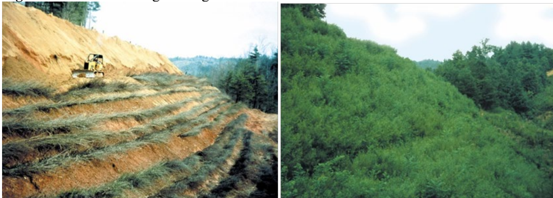
Left photo at installation and right photo was taken 1 year after installation (Robbin B. Sotir & Associates photos)
