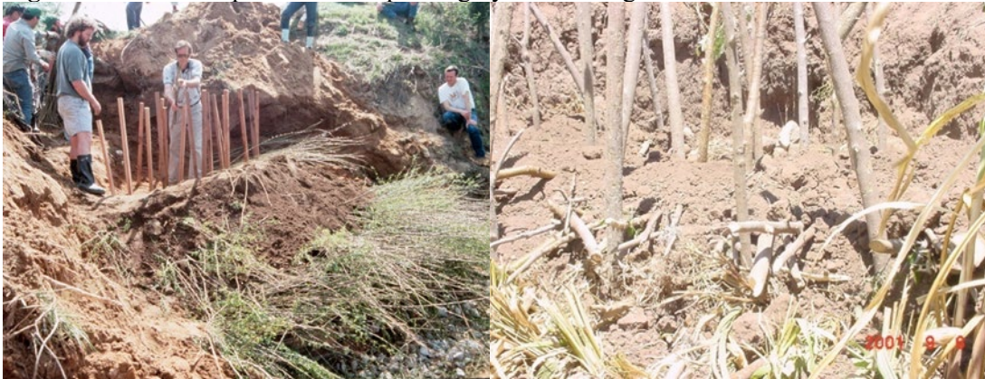
Photo on left uses timber poles. Photo on right uses live poles
