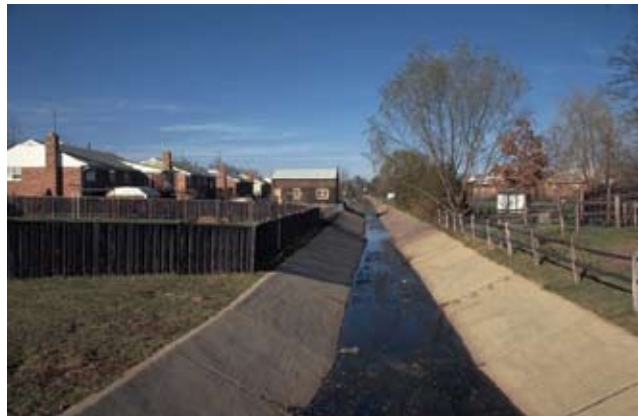
Figure 4-3 Lined channels may be necessary, based on boundary constraints, drainage needs (discharge capacity), and maintenance costs.
