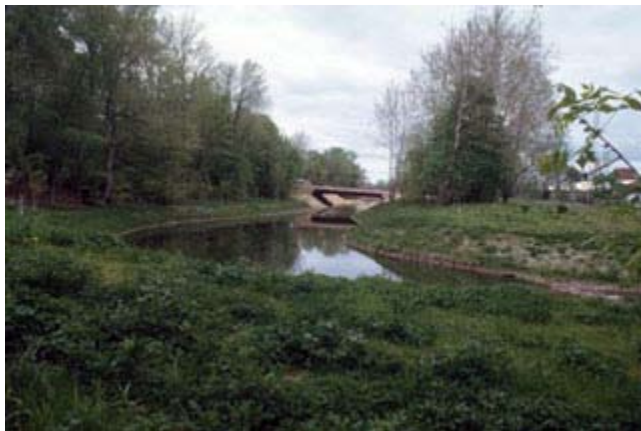
Figure TS14L-22 ACB revetment system 1 year after completion ( Photo courtesy of Joe Polulech )
