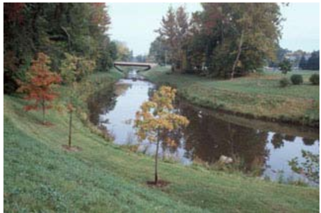
Figure TS14L-23 ACB revetment system 2 years after completion ( Photo courtesy of Joe Polulech )
