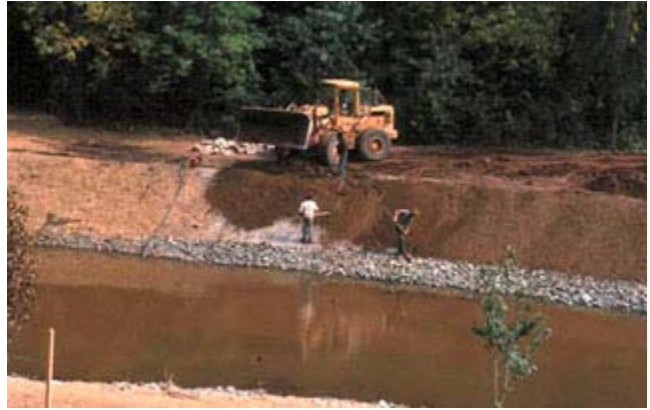
Figure TS14L-21 Filling ACBs with top soil ( Photo courtesy of Joe Polulech )
