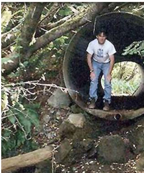
Figure TS14N-18 A significantly perched culvert (Photo courtesy of Dick Quinn, USFWS, Newton, MA)
