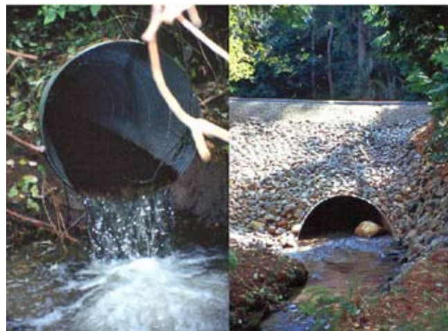
Figure TS14N-24 Undersized perched culvert (left) replaced with larger pipe designed using stream simulation option
