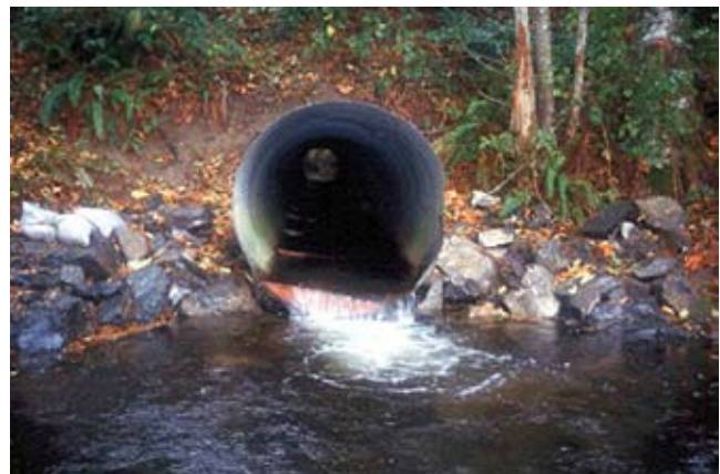
Figure TS14N-21 Round, corrugated metal culvert retrofitted with corner baffles to improve fish passage
