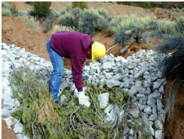
Figure TS14P-24 Rock and brush dam under construction in AZ (Photo courtesy of Pete Bautista)
