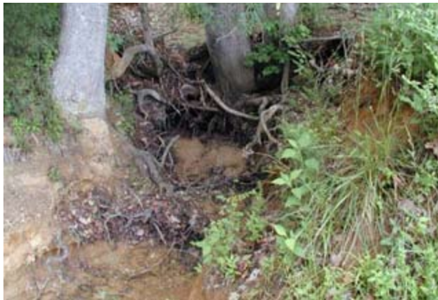
Figure TS14P-5 Headcut halted by tree roots in Union County, SC
