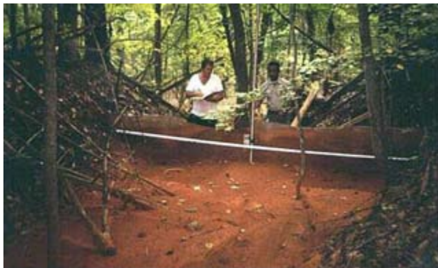
Figure TS14P-13 Erosion resulted in sediment from a small gully trapped in filter fabric fence
