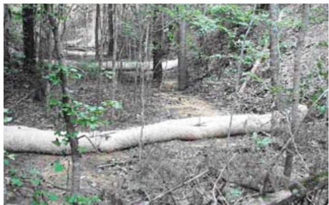
Figure TS14P-19 Coir logs used to complement surface stabilization and revegetation measures used in background gully channel
