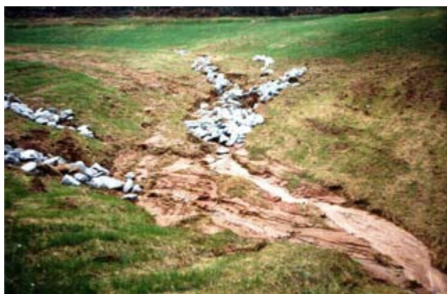
Figure TS14P-33 Rock placed in gullies arms the flow path on steeper slopes to prevent gully advance
