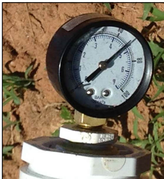
Figure SC6-33a Non-filled pressure gauge showing 70 psi downstream of the zone control unit
