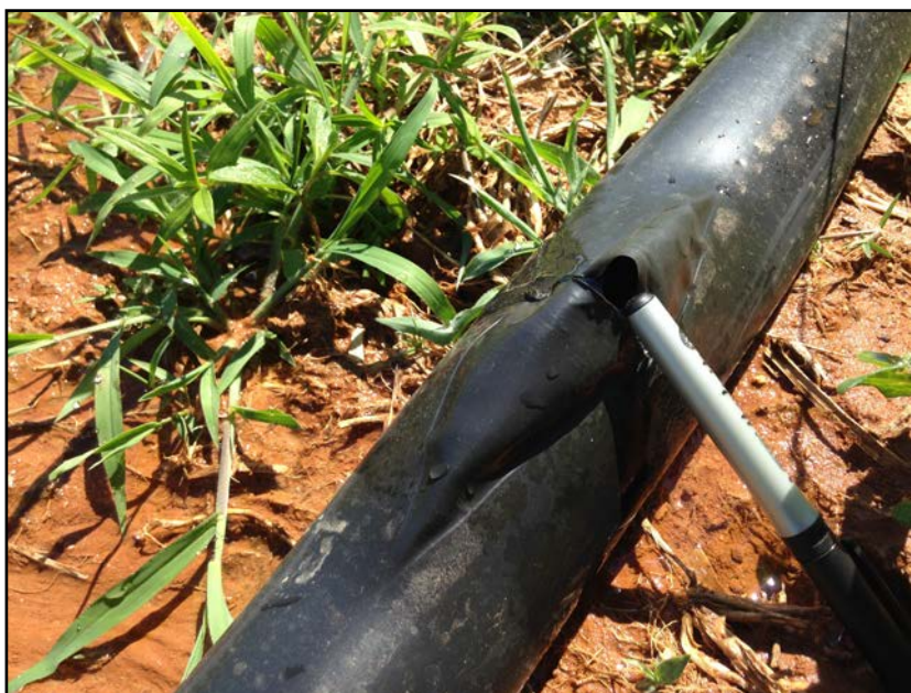
Figure SC6-34a 2 inch PE (Oval) hose "burst" due to PRV flow range outside of zone flow rate (gpm)
