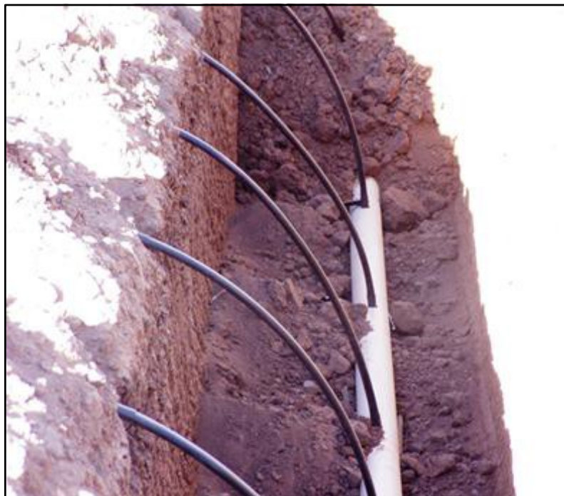
Figure SC6–39 SDI submain with flexible feeder lines connected to the buried drip tape
