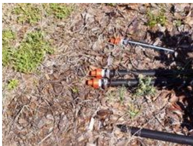
Figure 7–90 Example of end of line flushing valves
