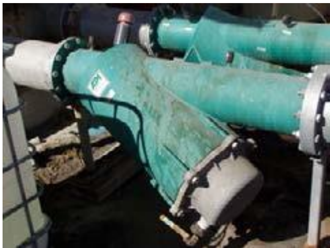
Figure 7–28 A large-diameter, steel, in-line screen filter
