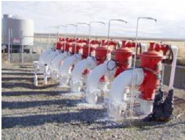
Figure 7–29 A battery of automatic flushing screen filters
