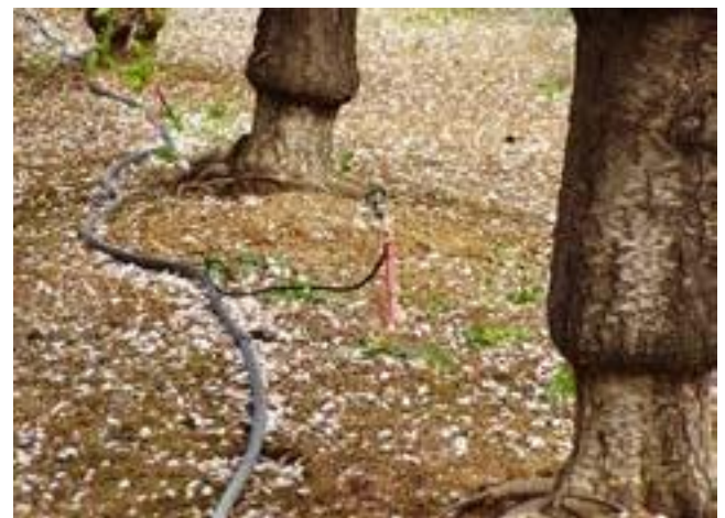
Figure 7–62 A microsprinkler system in an almond orchard
