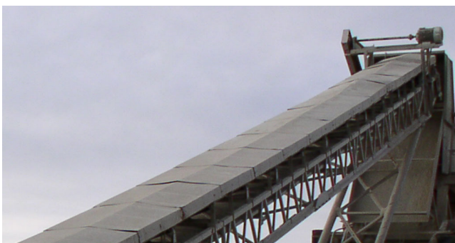
Figure 13-6 Covered conveyor belts
