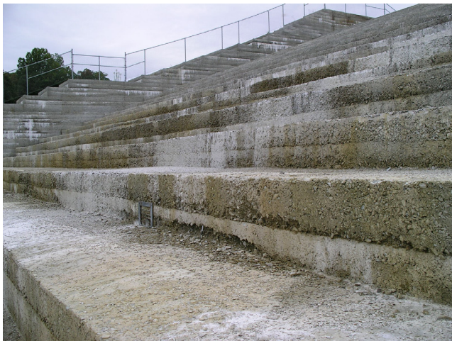
Figure 13–9 Rock pockets in the finished surface
