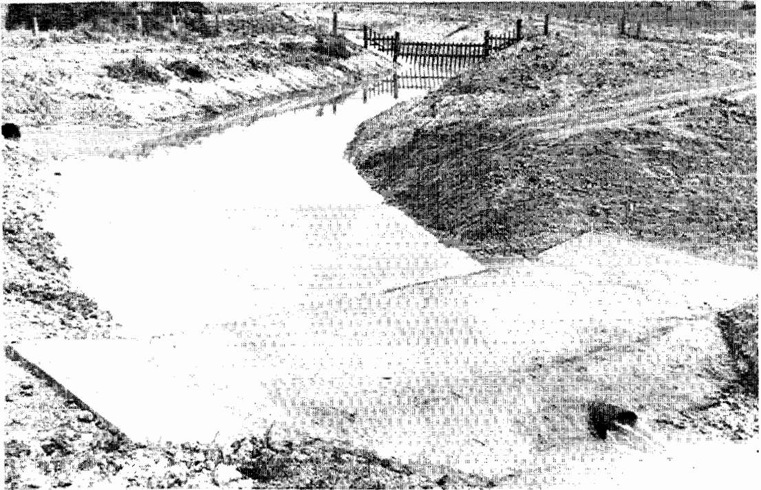
Low water crossing, watergate and pipe drop
